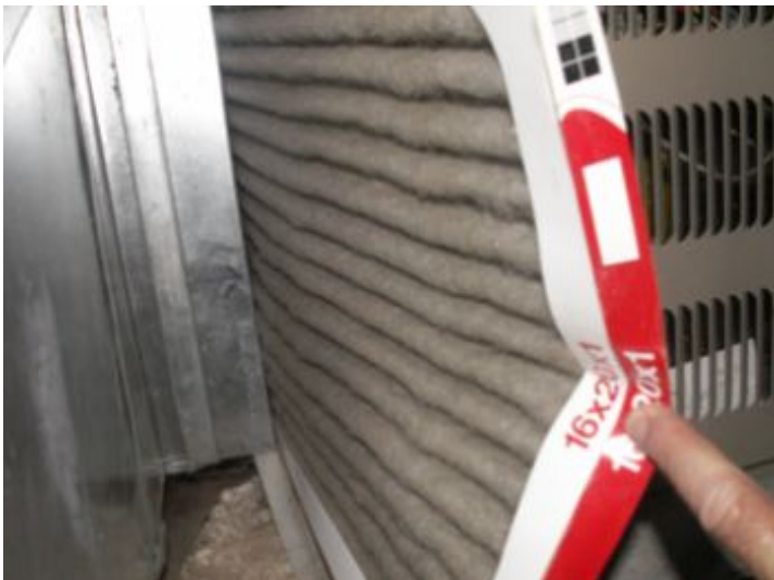
Furnace filter clean.
