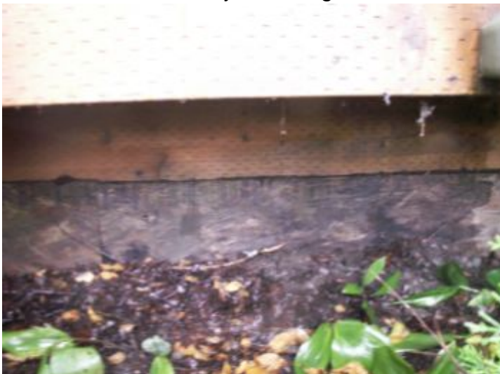
Below front deck. OSB sheathing in contact with the ground.
