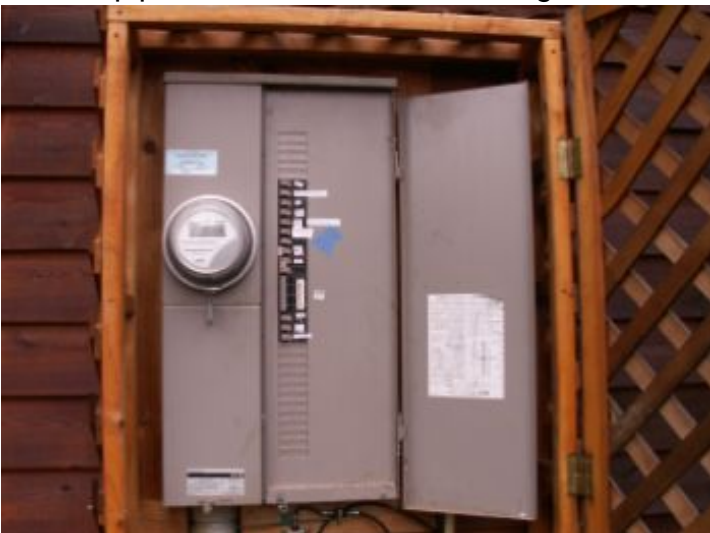
Electrical main and breaker panel. Labeled. No deficiencies observed.
