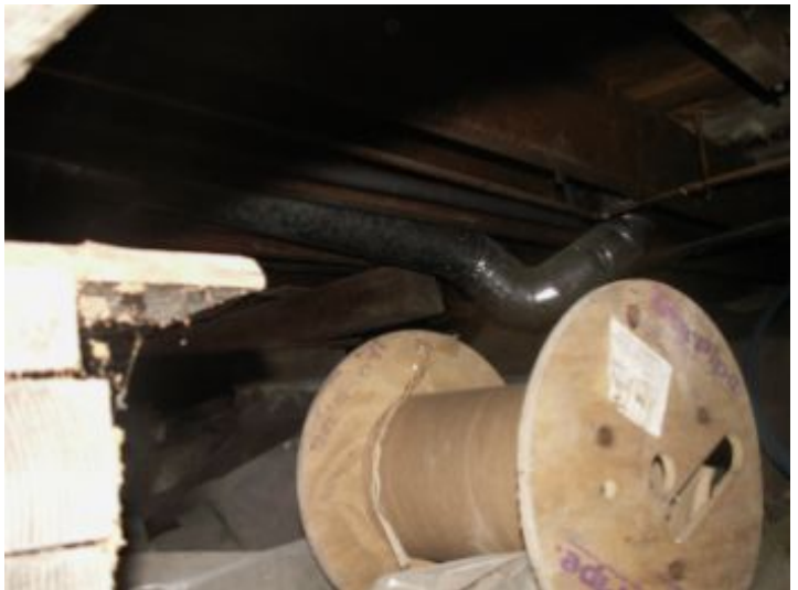
Debris left in crawlspace.
