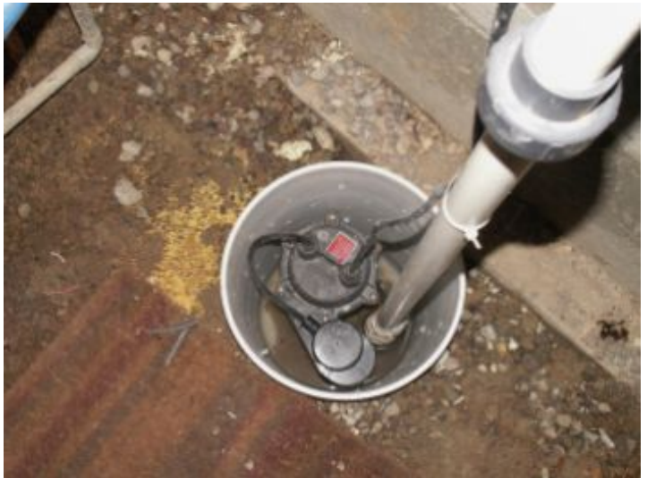
Sump pump in mechanical crawlspace functioning. No deficiencies observed.
