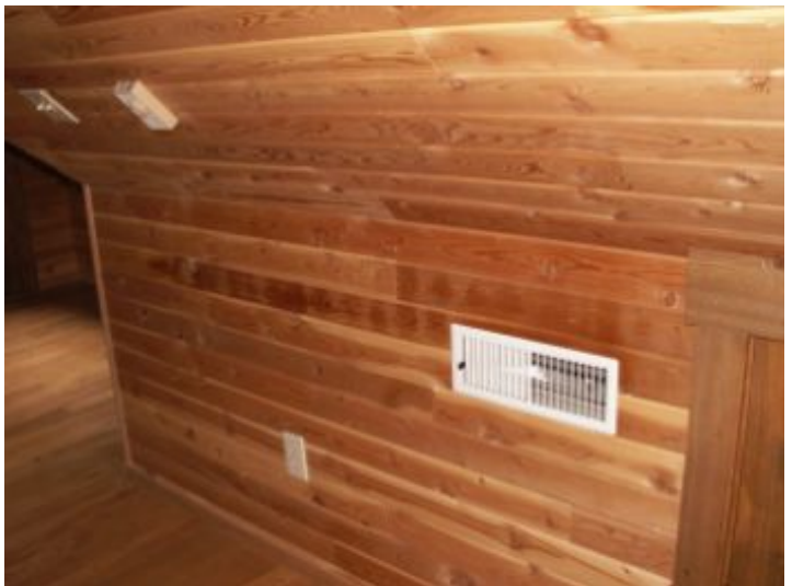
Loft exhaust fan. No deficiencies observed.
