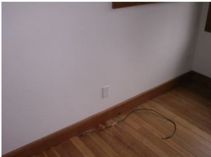
Living room outlet with an open ground.
