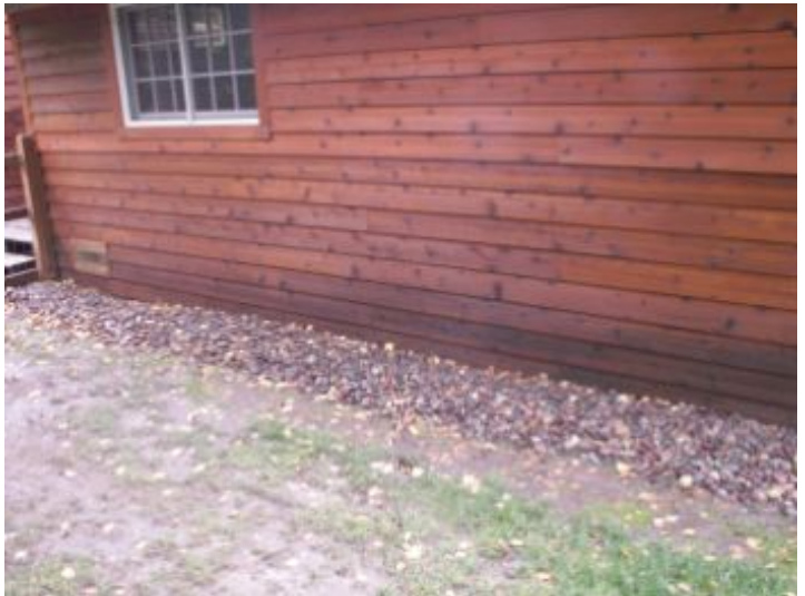
Grade on west side of house is sloped toward the house. Gravel is used to prevent mud splashing on to siding.
