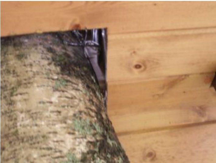
Front porch roof. Birch tree trunks in contact with roof framing.
