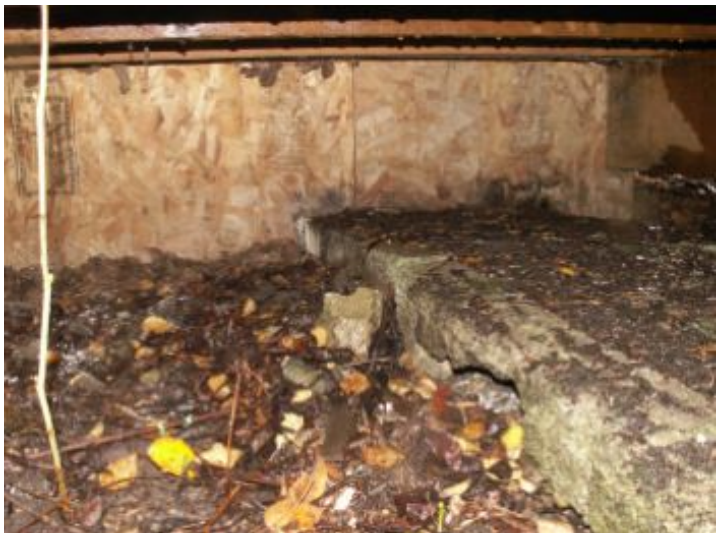
Below deck at front entry. OSB sheathing in contact with ground.
