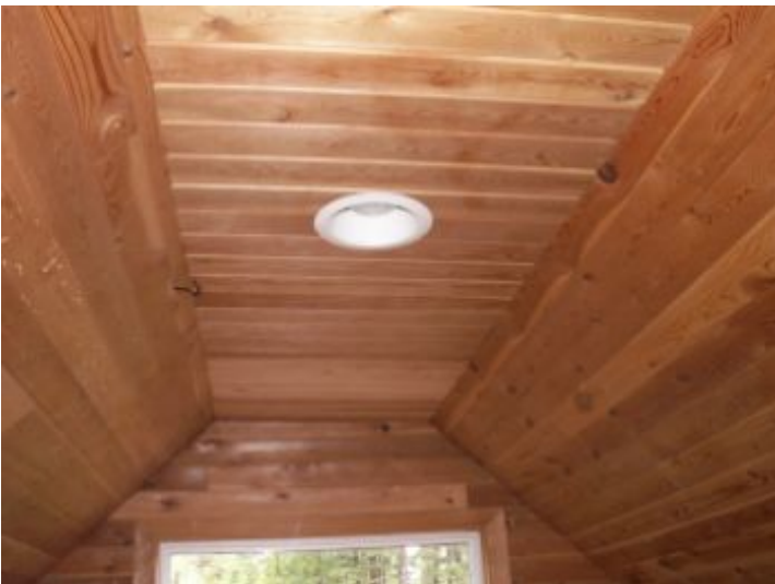
Loft fixture did not operate. Replace bulb and re-check.
