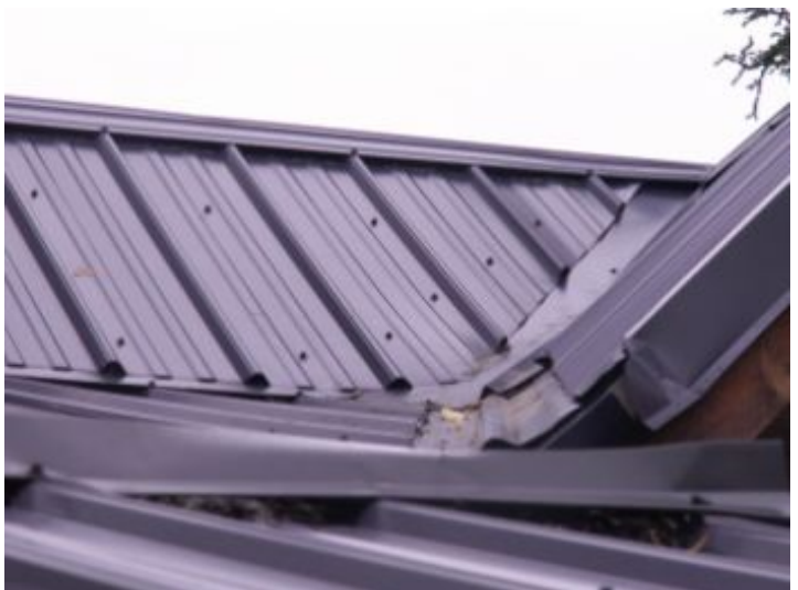
Snow stop is damaged but functioning. Cosmetic issue.
