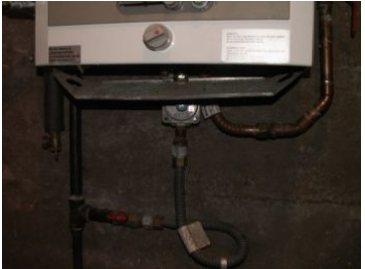
On Demand Water Heater in mechanical crawlspace. No deficiencies observed.
