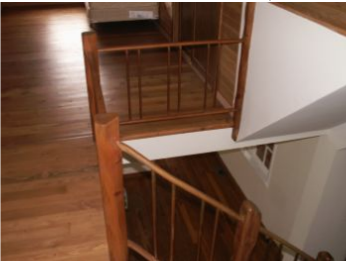
Loft/stair railing at 26 inches. Code minimum is 36 inches for loft and 34 inches on stairs.
