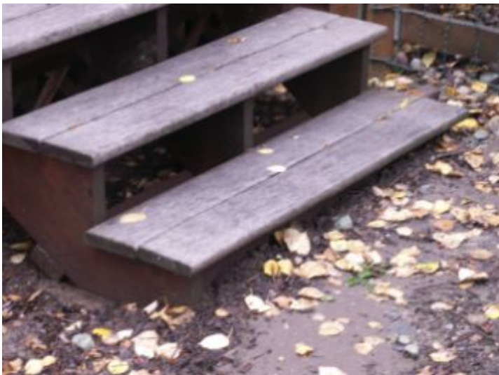
Stair stringers in contact with dirt. Contact with dirt will accelerate deterioration.
