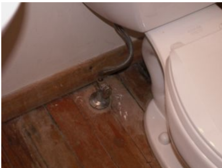
Bathroom floor with evidence of previous leaking. Not leaking currently. Monitor.
