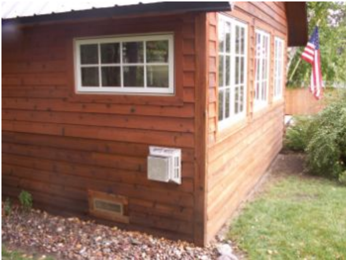
Gas stove exhaust vent below an operable window. Does not meet current codes and standards.
