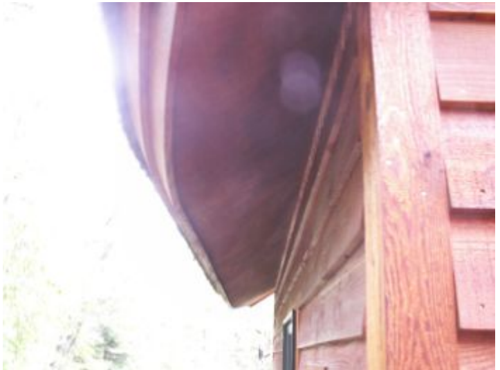
No soffit venting present in the bunkhouse. May not be needed depending on type of insulation.
