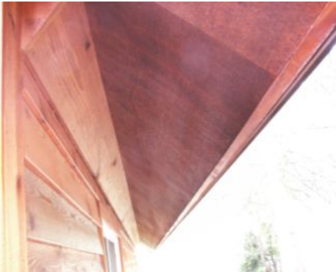
No soffit venting present. May not be needed depending on type of insulation in the roof.
