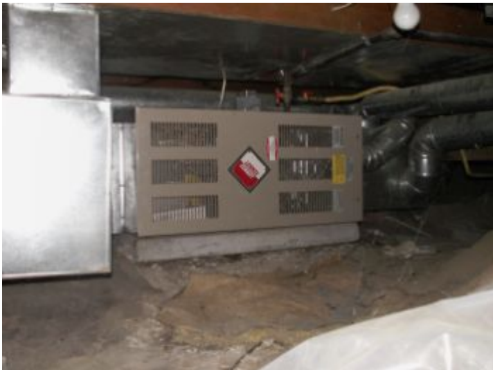
Crawlspace. Gas furnace. No deficiencies observed.
