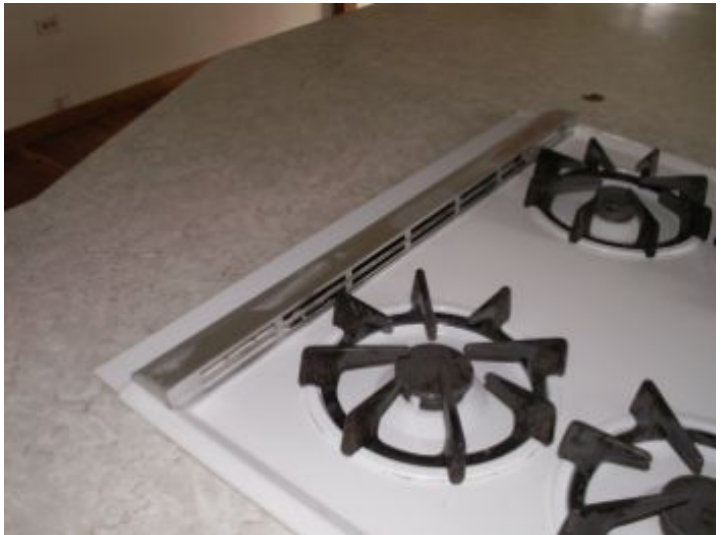
Range exhaust fan does not operate.
