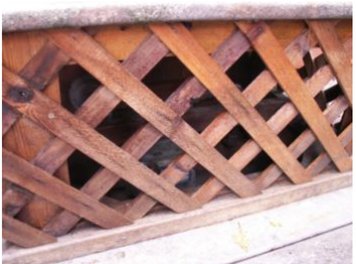
Location of gas meter. Below rear deck.
