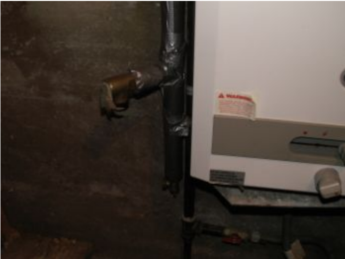
TPR valve on On Demand Water Heater should be piped to within 6 inches of the ground.
