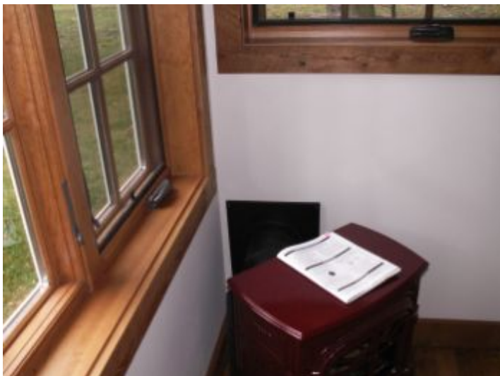
Gas exhausts below an operable window. Does not meet current codes and standards.
